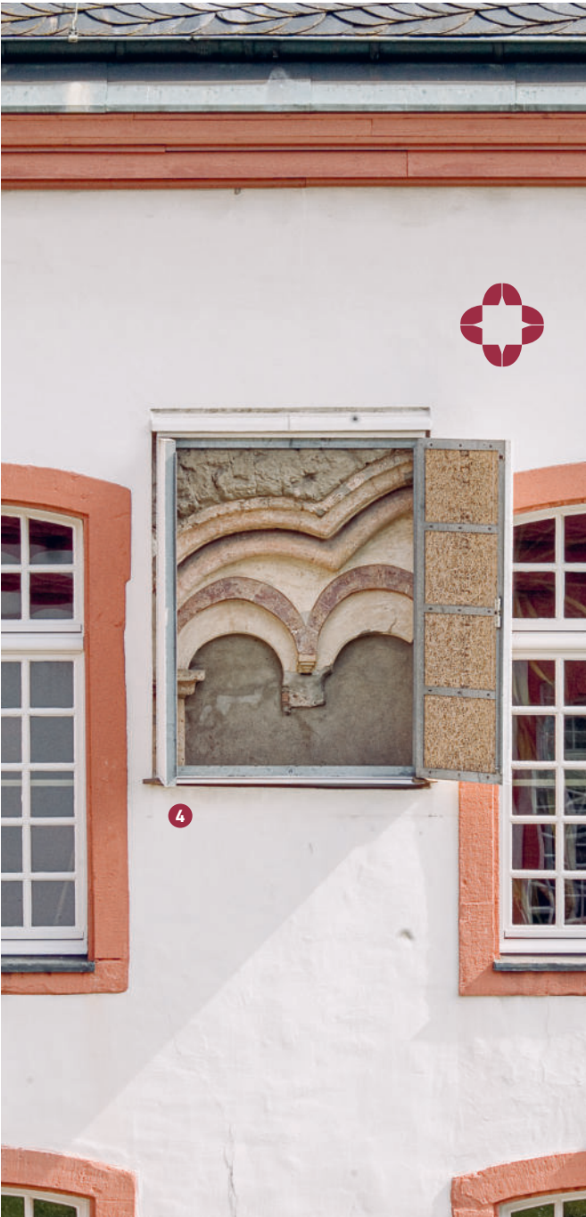
The east wing of the prelatore was originally the front of the medieval monastery building. The Romanesque construction can still be seen under the Baroque façade through a window.
